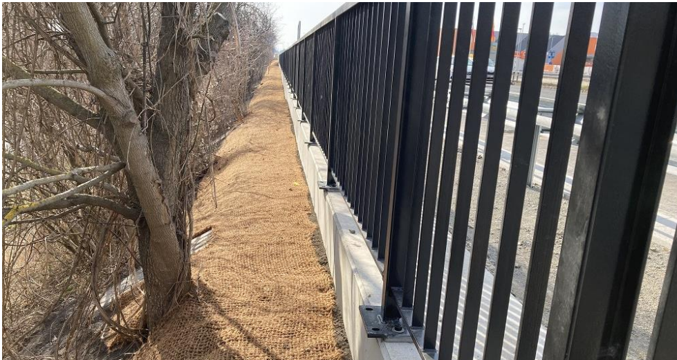
Caption: The slopes have been modified, including a new retaining wall, which has allowed the widening. (© PORR)
