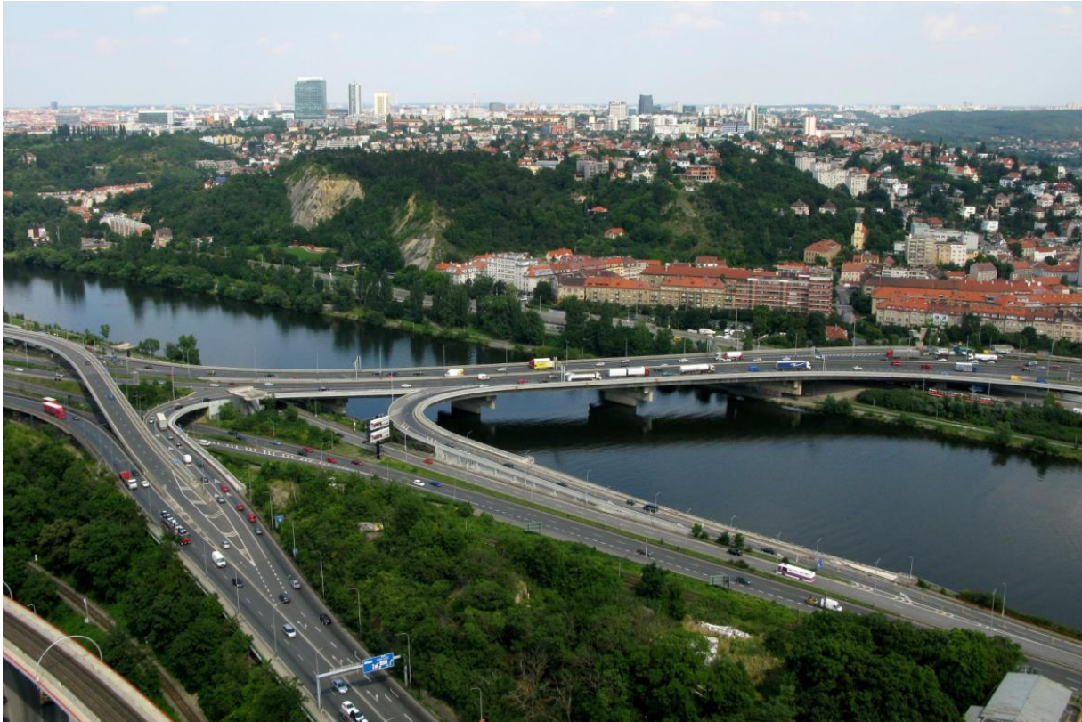
Caption: In 2022, PORR will work on the right half of the southern part of the bridge in the direction from Smíchov to Jižní spojka and on the Strakonická ramp. (© TSK Praha)
