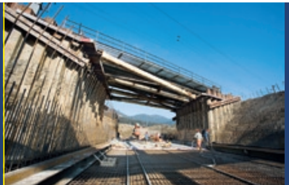
The project B 170 Brixen bypass in Tyrol includes the construction of the underground route, operational buildings, water protection facilities, emergency exits and emergency stairs.
