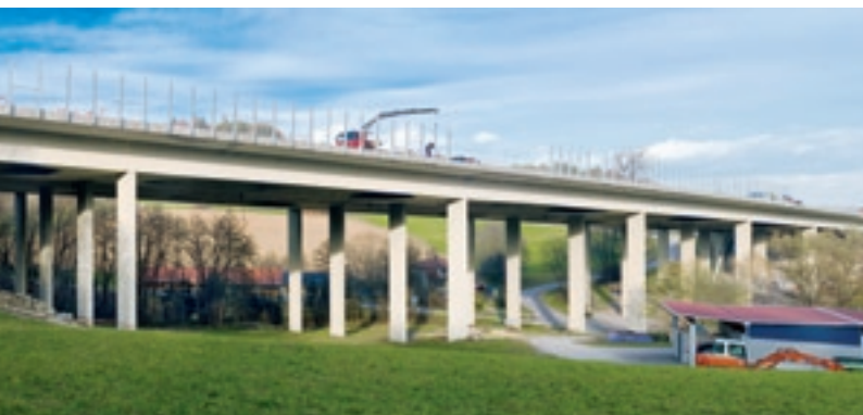
Road and bridge repair work was carried out on the A 2 Südautobahn, Gleisdorf West – Lassnitzhöhe . This includes renovation of the edge beams, structural insulation, slope and concrete reinforcement.
