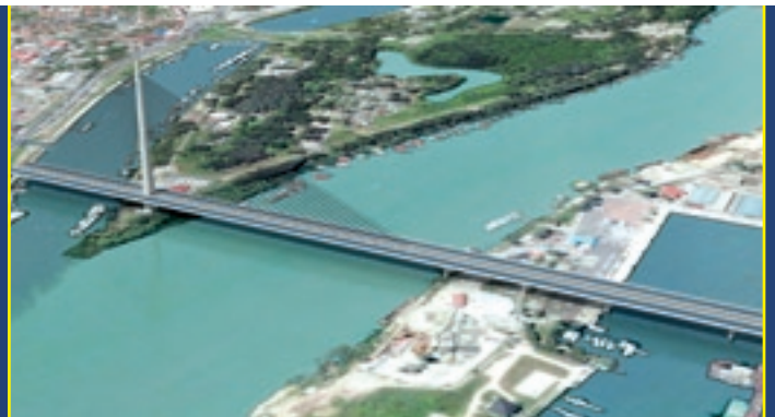
A 929 m-long cable-stayed bridge, the Sava Bridge , has been under construction in Belgrade, Serbia since May 2008. The bridge will be supported by a 200 m high pylon.
