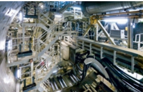
The project H3-4 Münster Wiesing in Tyrol includes the construction of a two-track railway tunnel, approx 5.800 m long. This will be executed mainly with the hydroshield tunneling method.
